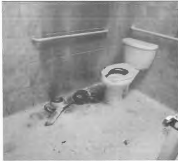
View of interior of handicapped men's bathroom stall at 10 Fitness with shadowing fire patterns visible on the tile wall where the toilet paper dispenser had previously been mounted.
