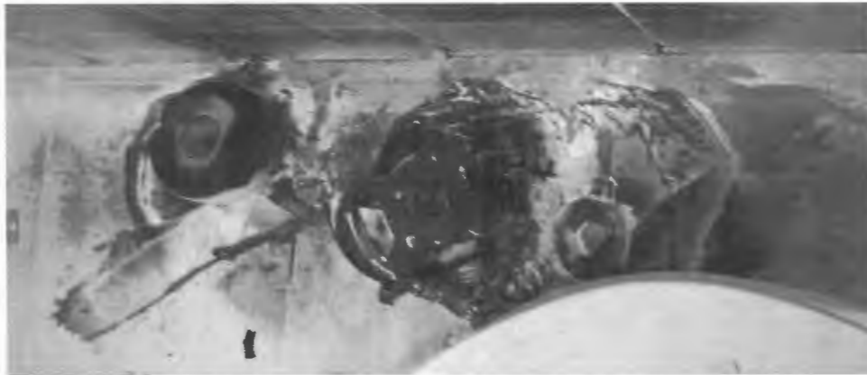
Closer view of fire damage to plastic dispenser and toilet paper rolls.
