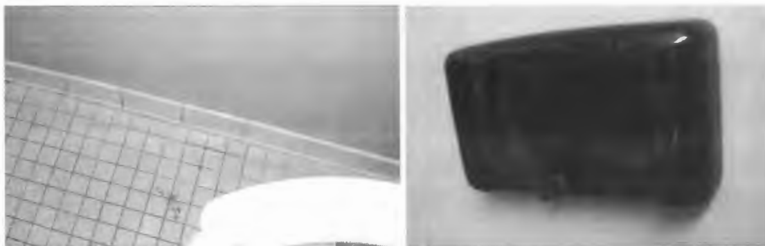
At left, remains of charred toilet paper on floor beneath wall-mounted toilet paper dispenser; at right, intact exterior housing of toilet paper dispenser.
